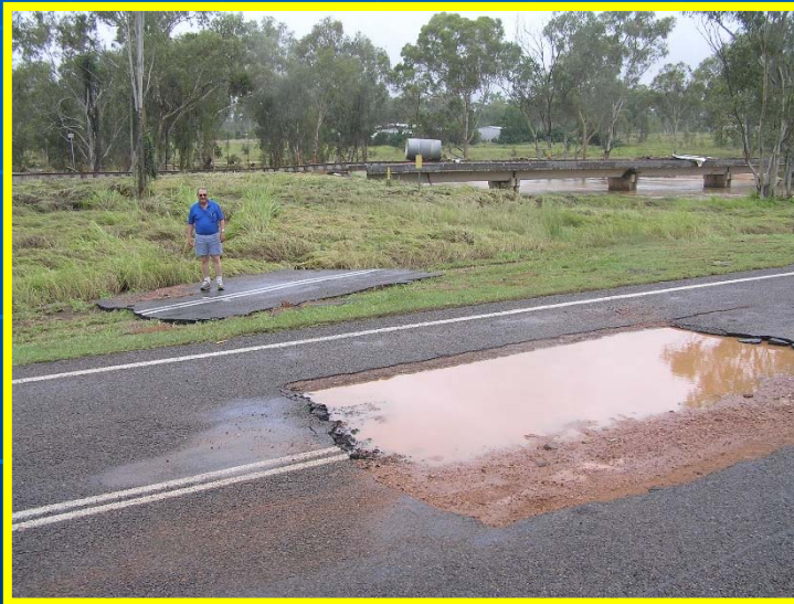
Damaged to Road Surface
